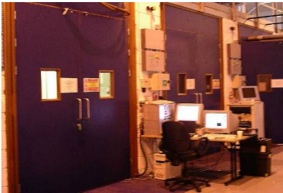
Figure 12: Motor testing cell (behind closed doors) with monitoring equipment
